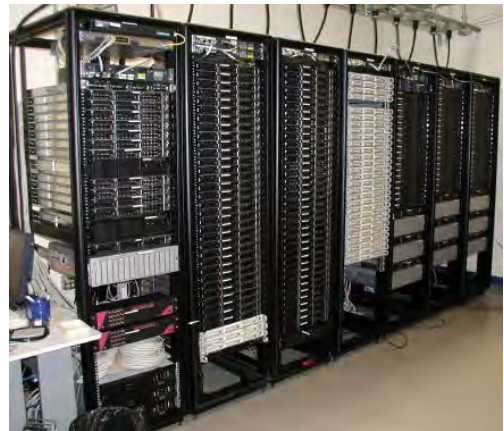
Figure 9: UW Tier-2 computing facility.
