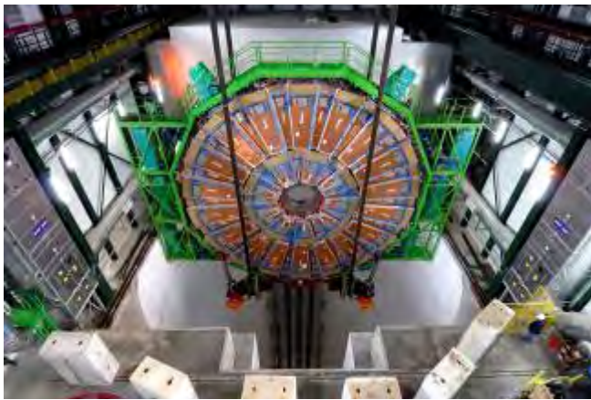
Figure 5. Disk YE+2 starting lowering into the 100 m shaft to the collision hall.
